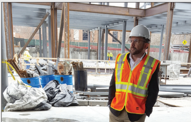
Gerald Hirsch, SHSMO senior associate executive director, surveys progress on the Center for Missouri Studies in April 2018. He now visits the site several times a week to ensure the project is executed as efficiently as possible.
