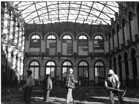
Workmen demolishing the trading hall ceiling, exposing its iron trusses and opening the grand room to the sky.
